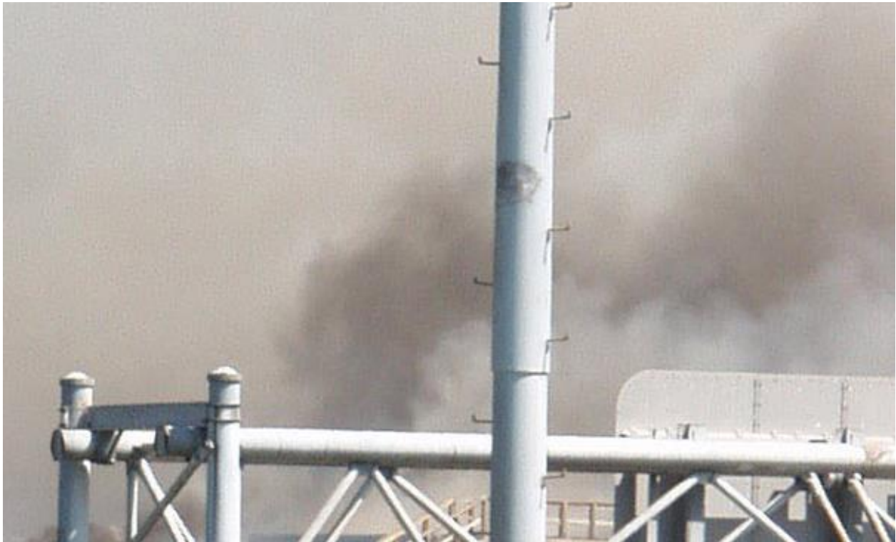
Figure 3 Detail view of scar and missing rung on the VDOT traffic camera pole cropped from the Coppage photo in Figure 1.
