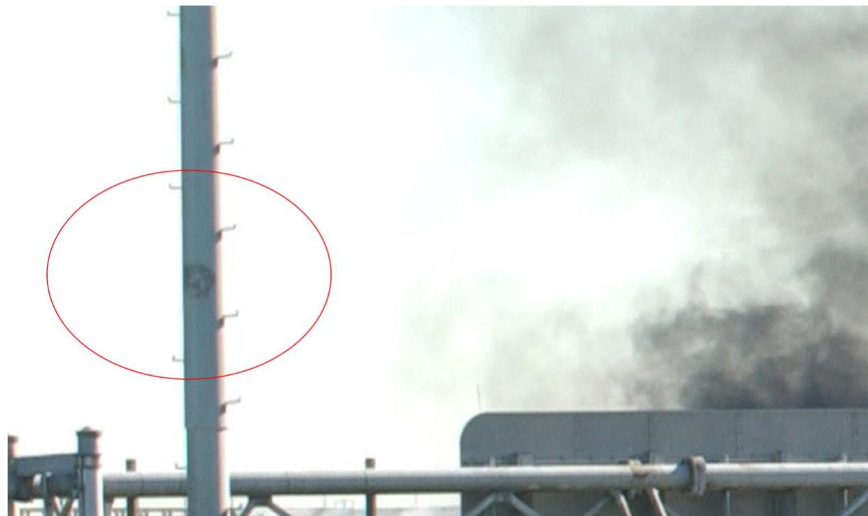
Figure 4 Confirming view from a different angle showing the rung to be missing, cropped from a Jason Ingersoll photograph taken earlier in the day before the Pentagon roof collapsed.
