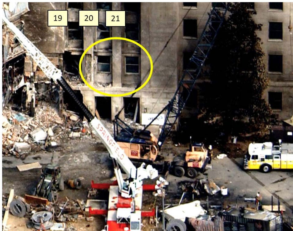
Figure 14: Debris on window sill between Columns 20 and 21.
