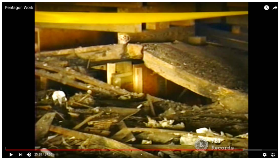
Figure 26: Uplifted second floor slab illustrating mechanical damage, not explosive detonations.
