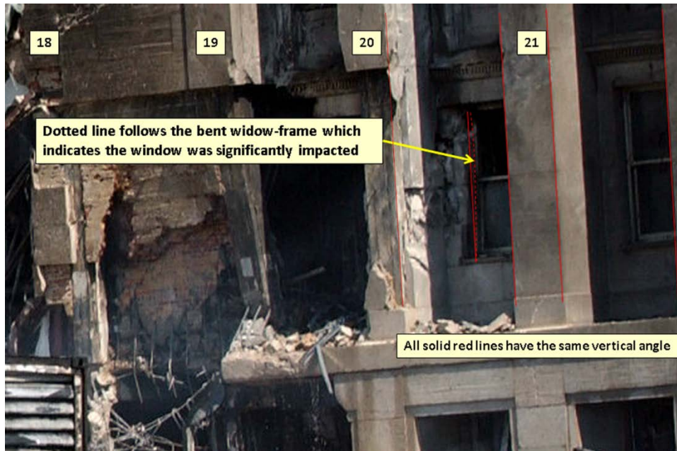
Figure 15: Bent window frame between Columns 20 and 21 with significant debris on the window sill.
