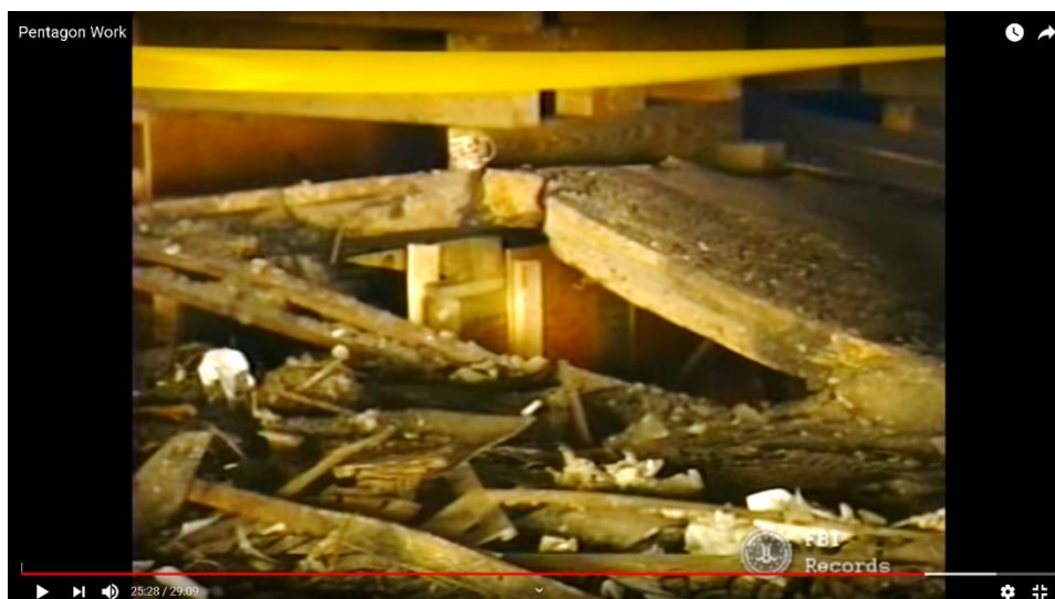
Figure 15: Uplifted Second Floor Slab illustrating mechanical damage, not explosive detonations.
