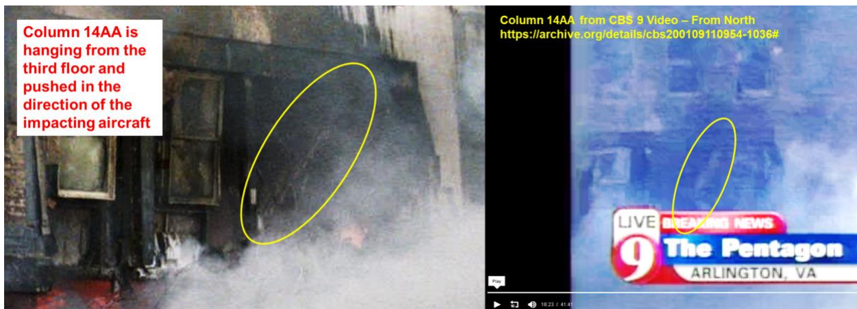
Figure 4: Column 14AA on the second floor is shown hanging from the third floor and pushed in the direction of the impacting aircraft.
