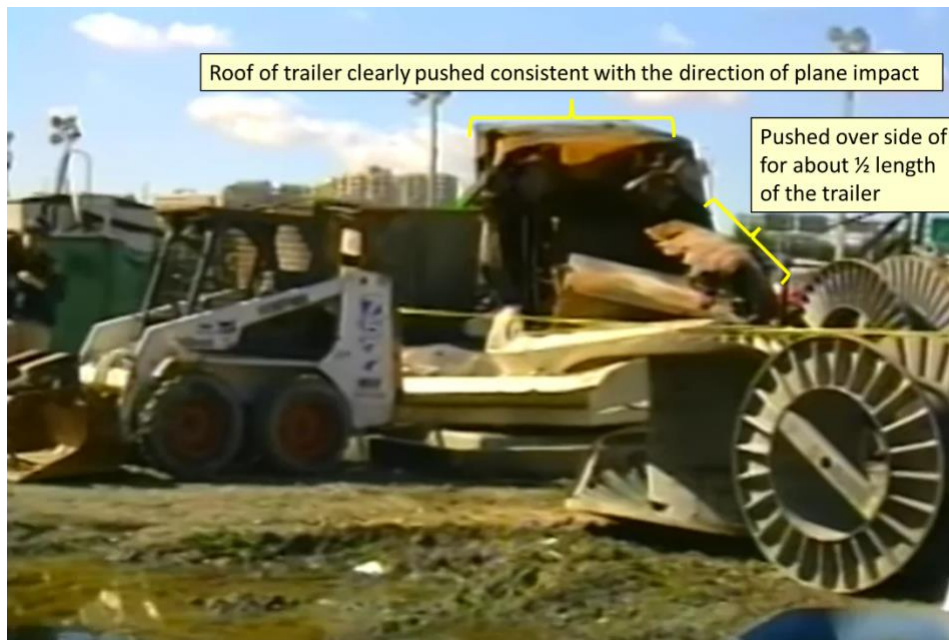
Figure 18: Ripped and pushed over covering of the generator with obvious distortion in direction of impact.
