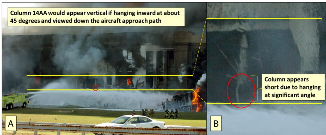
Figure 3: Column 14AA looks vertical when viewed from the approach angle, but is actually hanging and pushed in the direction of impact (left). The bottom of the column is fragmented (right) and clearly does not extend to the level of the second-floor slab.
