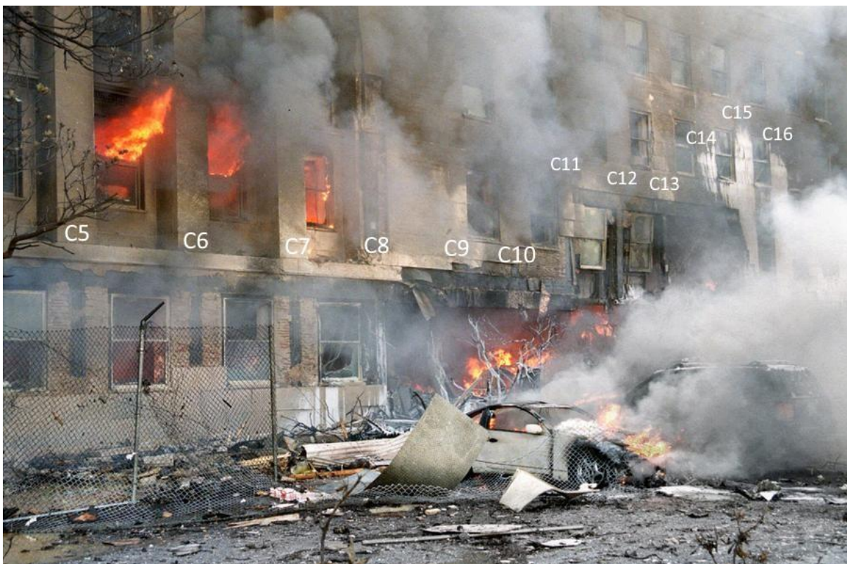
Figure 5: Left side of the entry hole on the Pentagon.
