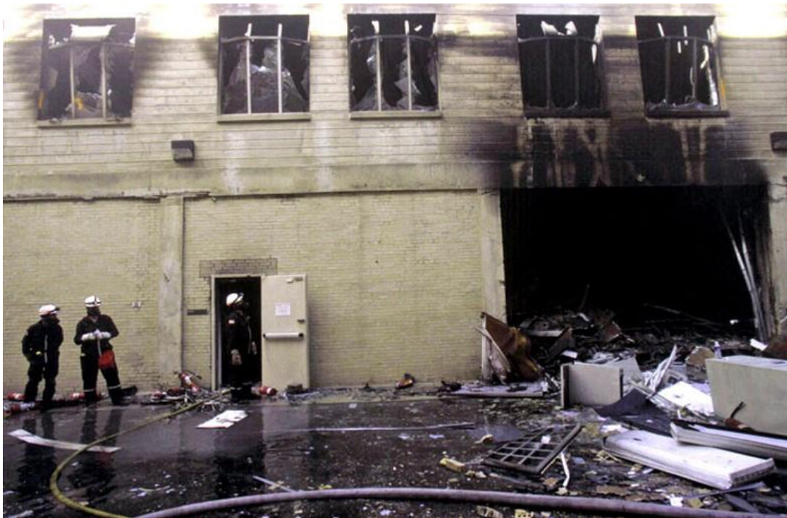
Figure 19: Damage in ring C between columns 5 and 10.
