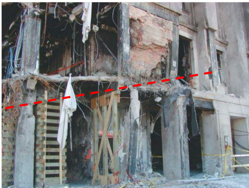
Figure 5.8 Facade damage to the south of the impact area
