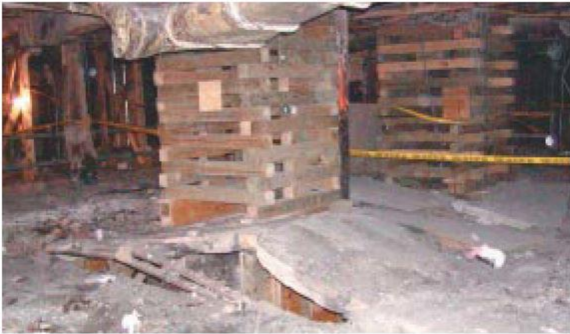
Figure 5.27 Breached second-floor slab
