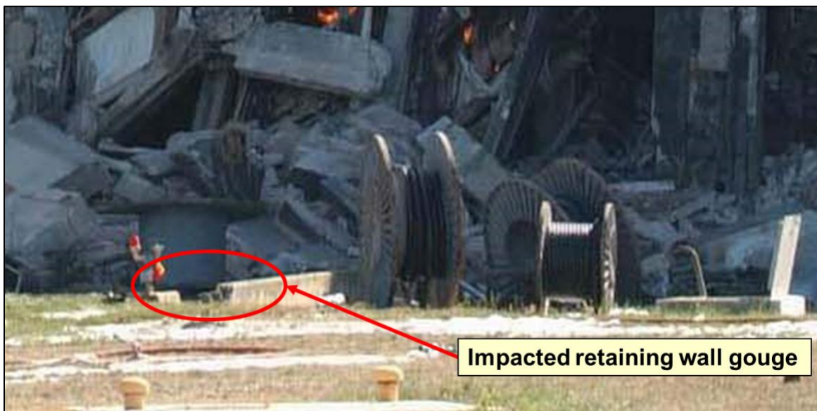
Figure 13: Gouged retaining wall
