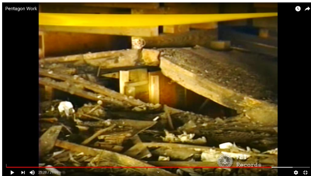
Figure 1: Uplifted slab is cleanly split along a single straight crack 1 .
