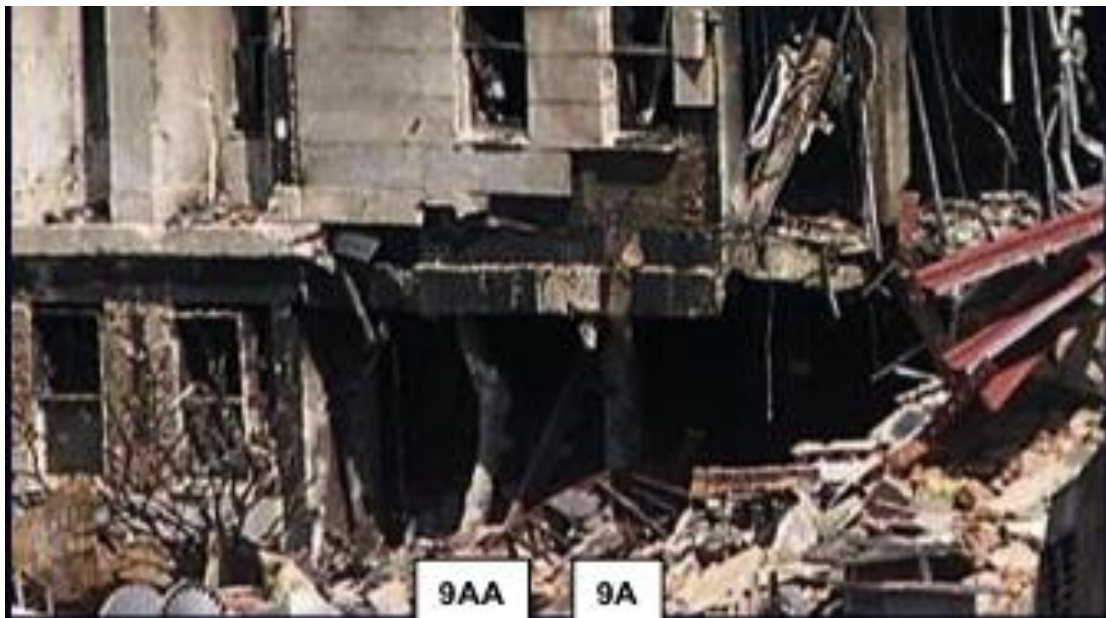
Figure 3: The inward bowing of column 9AA is a clear sign of impact.
