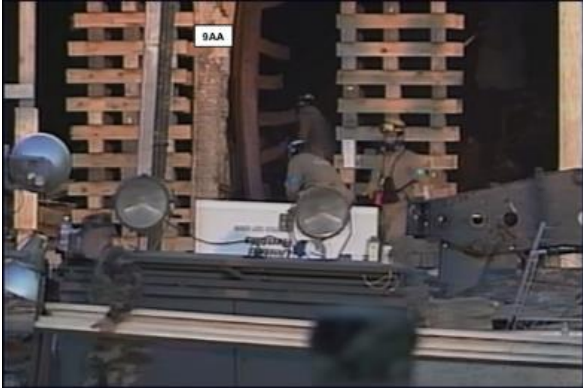
Figure 4: Note the steel "fingers" attached to the 8-inch square steel tubing. These originally pointed outward toward the lawn to hold a heavy blast-resistant window.
