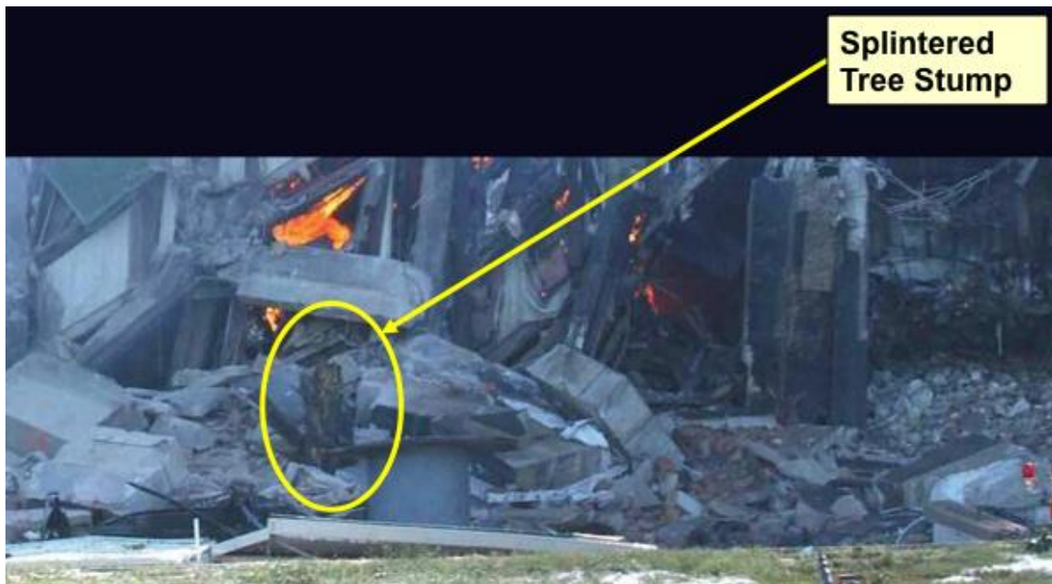
Figure 13: The stump from the tree in front of Column 16 shows that the trunk was literally torn off.
