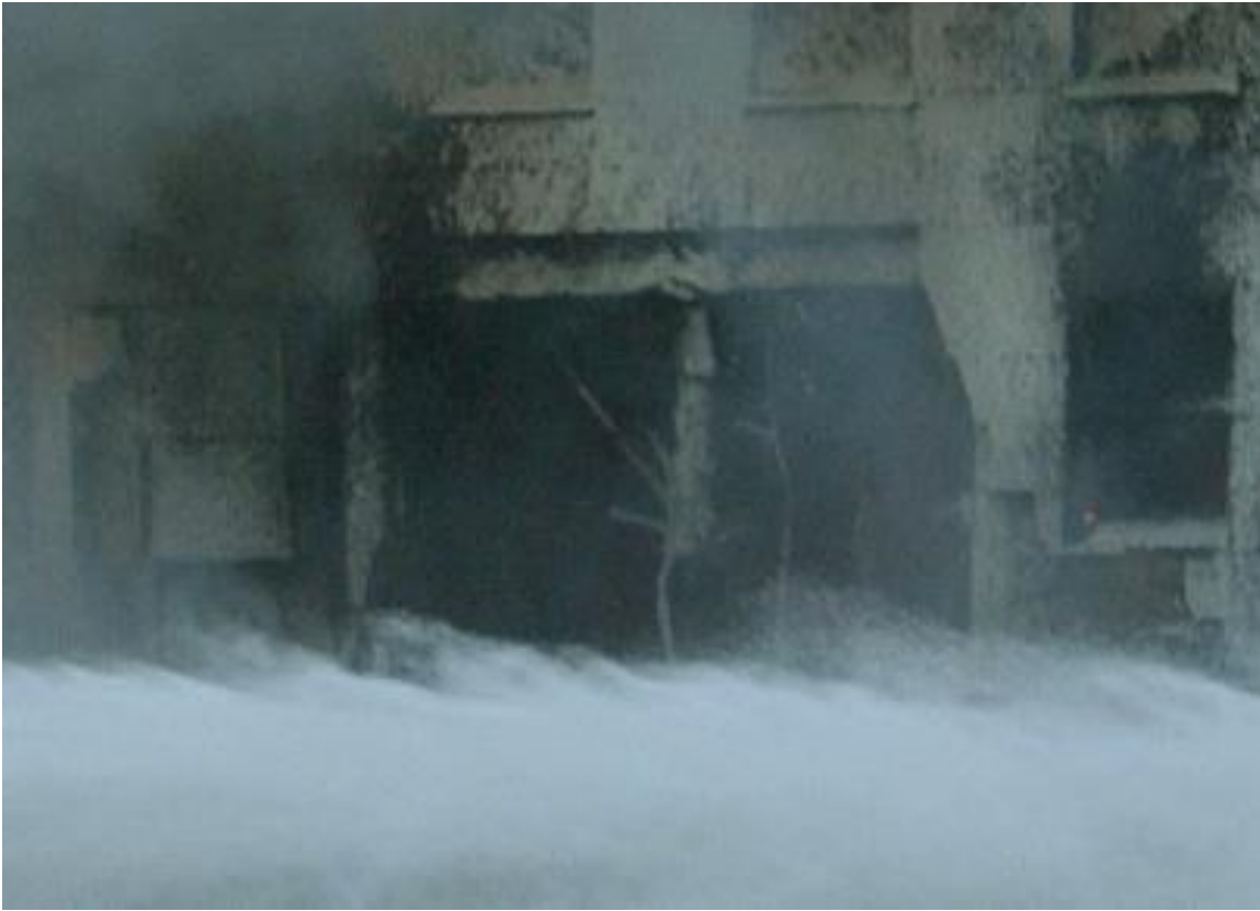
Figure 6: The highly misleading "small opening in the wall" at Column 14 on the second floor.
