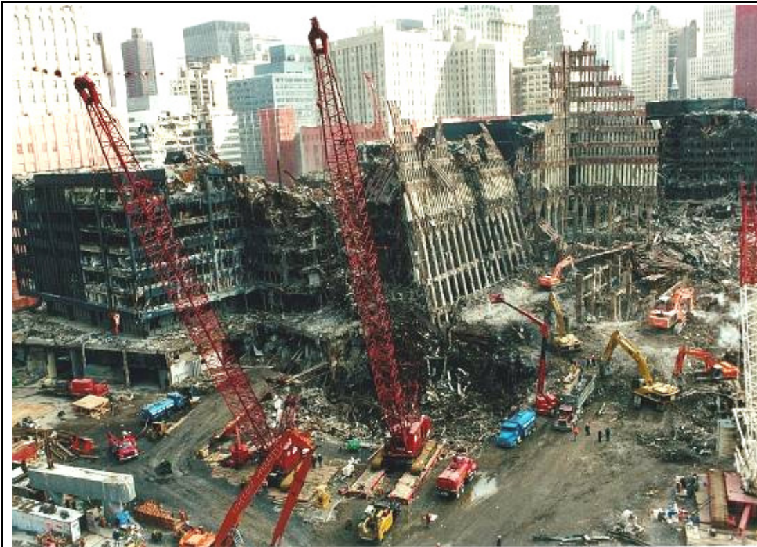
October 17, 2001: North tower. Much surface debris has been removed, but notice the compacted debris in the sublevels. 44
